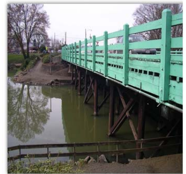
The City of Longview’s Washington Way Bridge Replacement project will replace the existing timber bridge with a concrete slab bridge, increasing the width to meet current design standards including sidewalk and curb.
